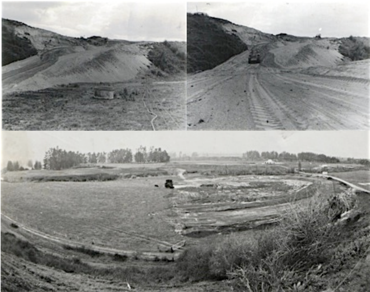
Top - The main entrance roadway into the property and the future exhibition area under construction. Bottom - Earthworks in the location known as Area One, later to also contain the Hamilton Car Club track.
